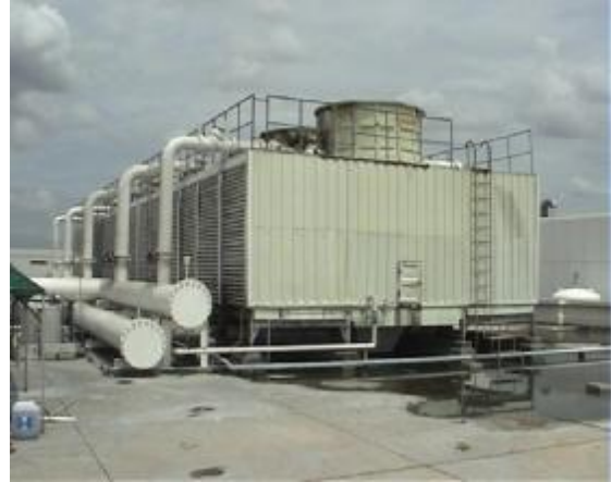
Cross Flow Cooling
