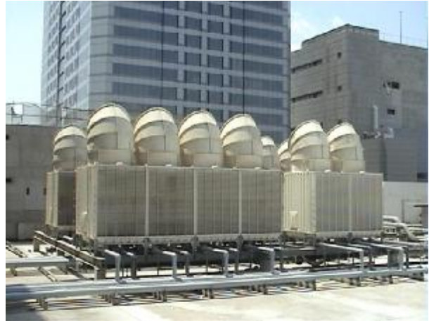
Cross Flow Cooling
